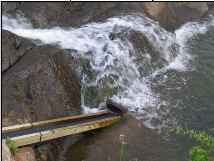
Photo 4: Experimental Eel Ramp Located at the Spillway of the Saluda Hydro Project
